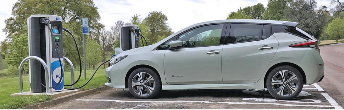
DC Fast Charging
